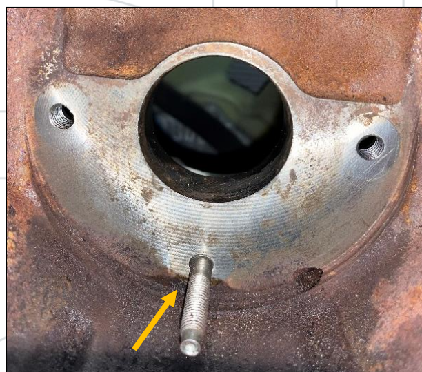
Figure 22: Pump Mounting Surface Cleanliness
